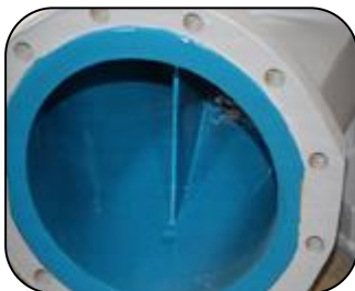
Salt water pump casing
